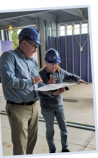
Lothian Skelton reviews blueprints with Andrew Young, VU Director of Architectural Services during a recent visit to campus.
